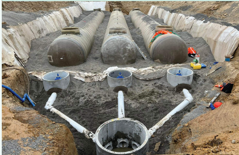
Sanson Wastewater Station
