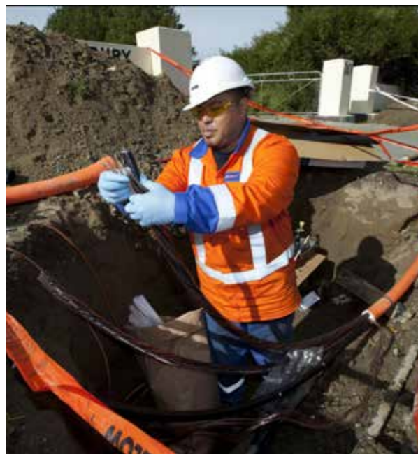
Underground the power lines along the main street
