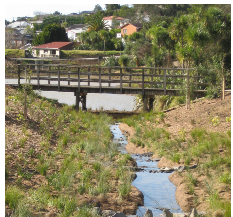
Examples show the network process - collection of stormwater at source - to rainwater tanks from roofs and to swales from roads, the direction of that runoff to a filtering area and then its discharge finally through a re-vegetated local stream to the receiving water course.
