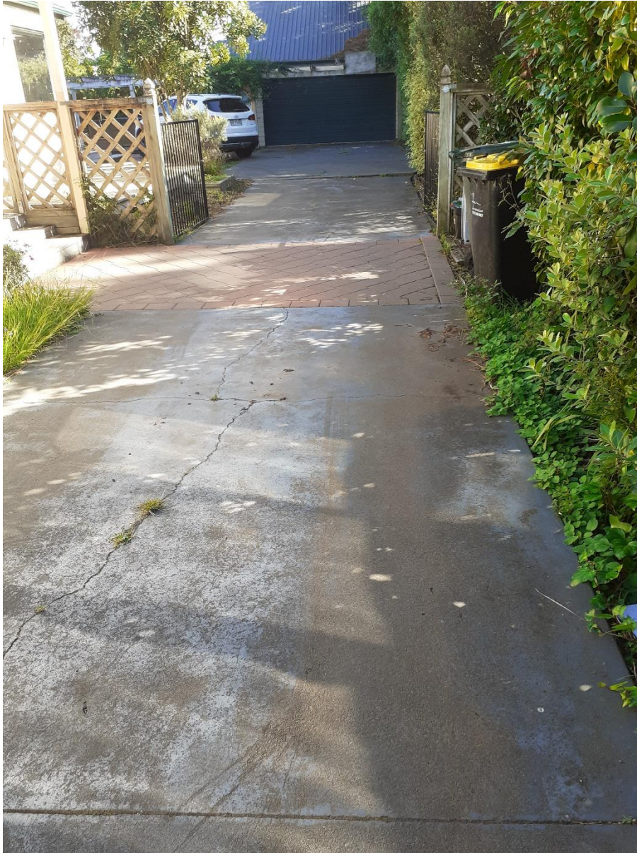
T6 Redwood – 26 Kimbolton Road. Note driveway cracks well away from tree with no upward deflection of surface
