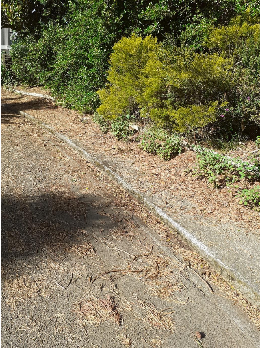
T6 – Pine Court next to tree. Note no damage to road, path or kerb caused by roots
