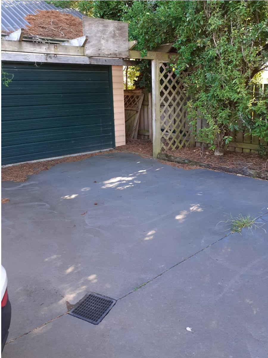
T6 Redwood 26 Kimbolton Road. Note concrete section closest to garage and tree is not cracked
