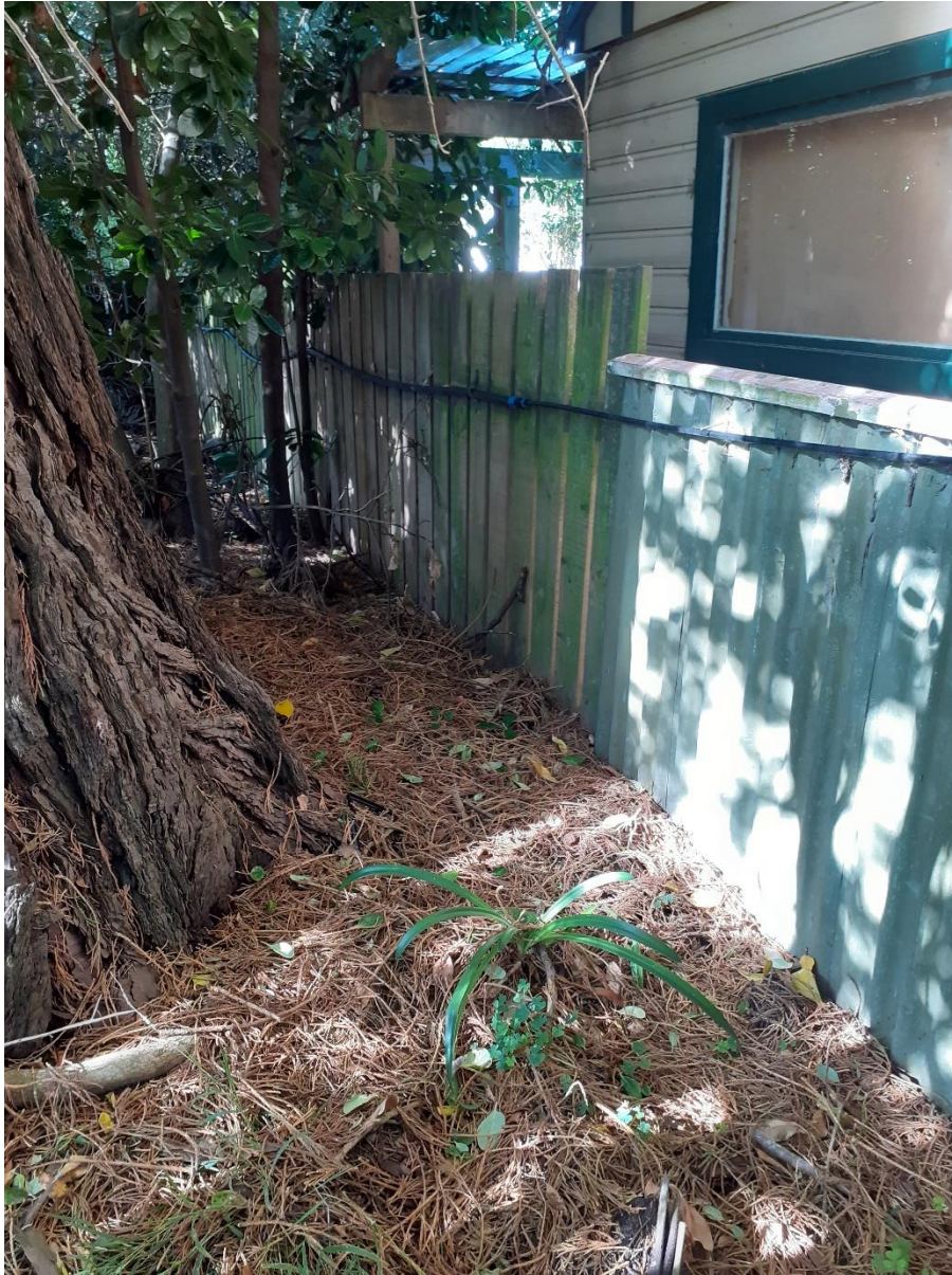
T6 Redwood – Position next to 26 Kimbolton Road. Note no damage to garage or fence caused by tree or roots
