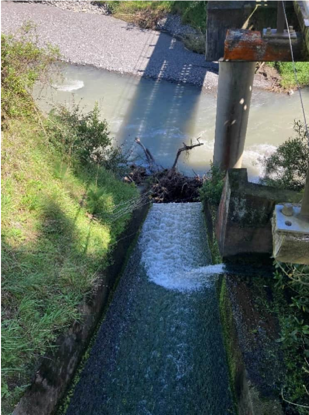
Figure 3.2: Photograph of concrete lined chute south of rail bridge over Tamaki River
