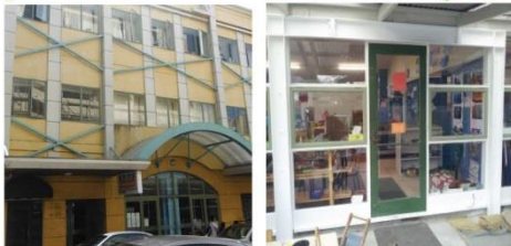
The two examples of external strengthening above contrast. The poor example (left) has cross braces (painted green) that run diagonally counter to the building's modulation. The good example (right) has a portal type bracing that fits with the door and window frame proportions and is painted the same principal white colour to de-emphasise it.
