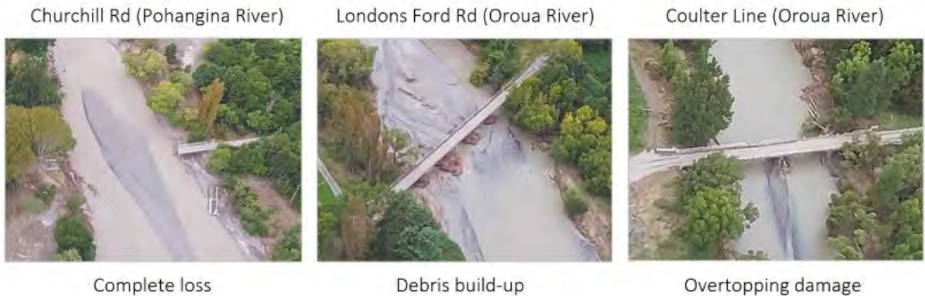
FIGURE 47: EXEMPLARS OF ADVERSE WEATHER EVENT DAMAGE
