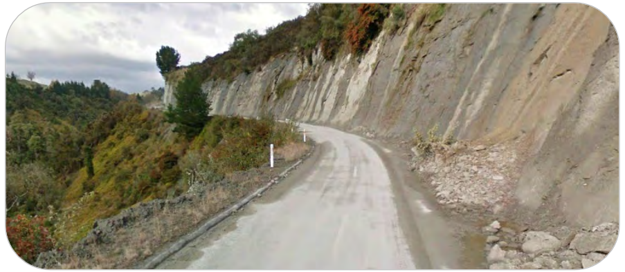
FIGURE 44: RUAHINE ROAD | FREQUENTLY OBSERVED CONDITION DUE TO SLIP ACTIVITY
