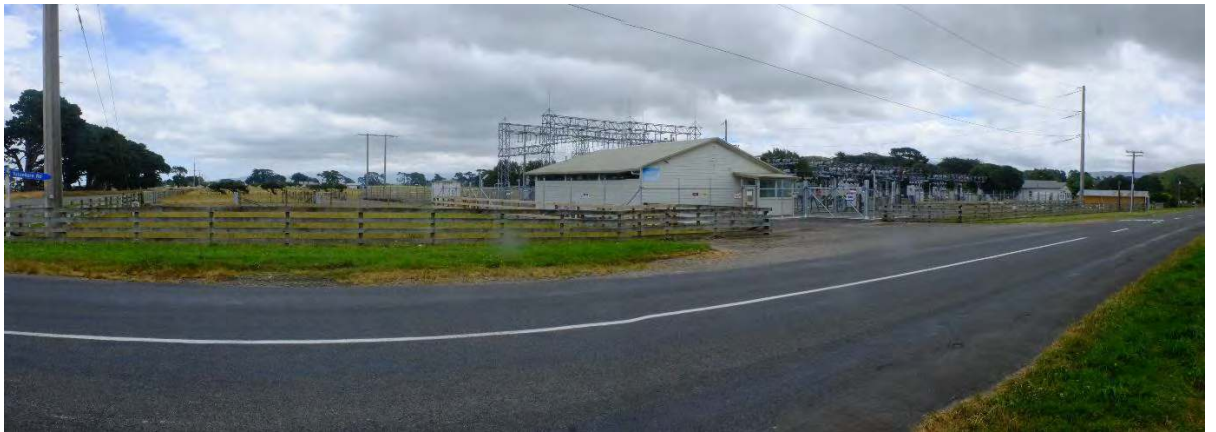
Fig 4: View of Mangamaire Substation from Tutaekara Road adjacent the facility travelling west.
