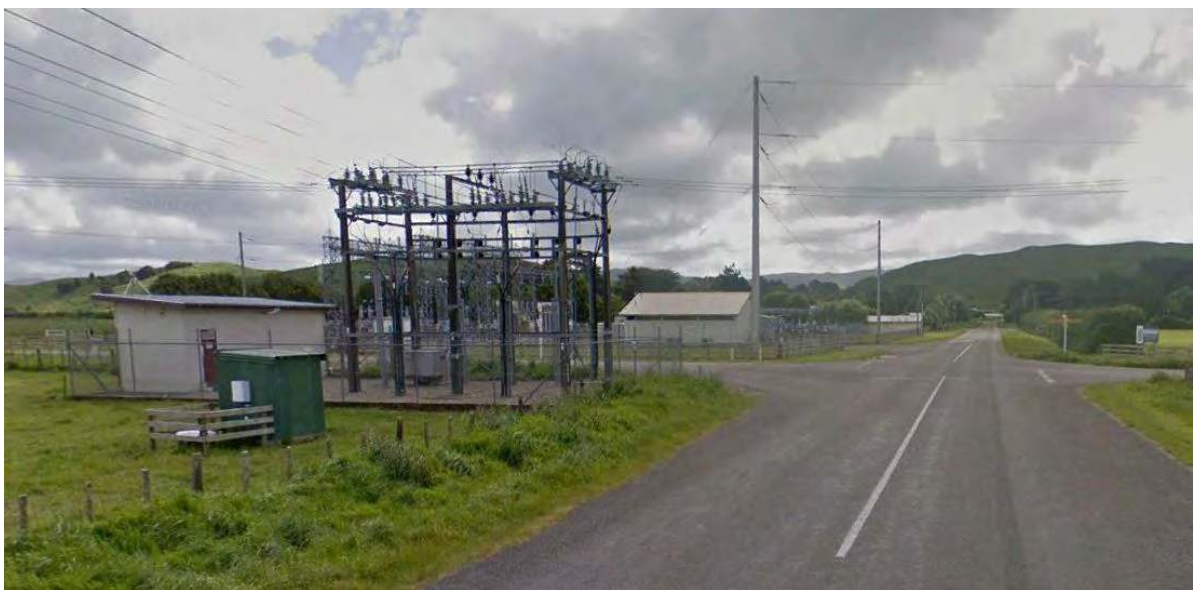
Fig 6: View of the facility on Tutaekara Road at the intersection with Mangamaire Road. The prominent facility extends across Mangamaire Road.
