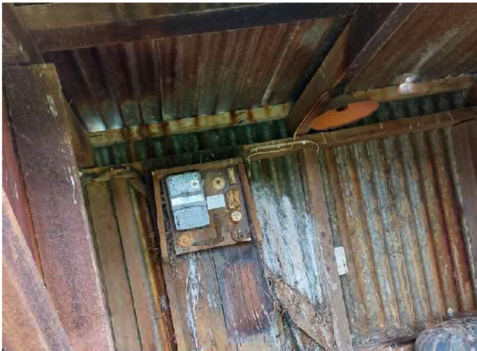
Plate D6: Interior of pump shed. Note the electrical distribution board.
