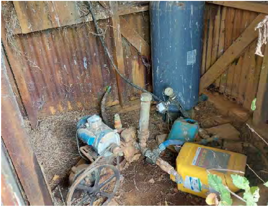
Plate D5: Interior of pump shed located north of former house site.
