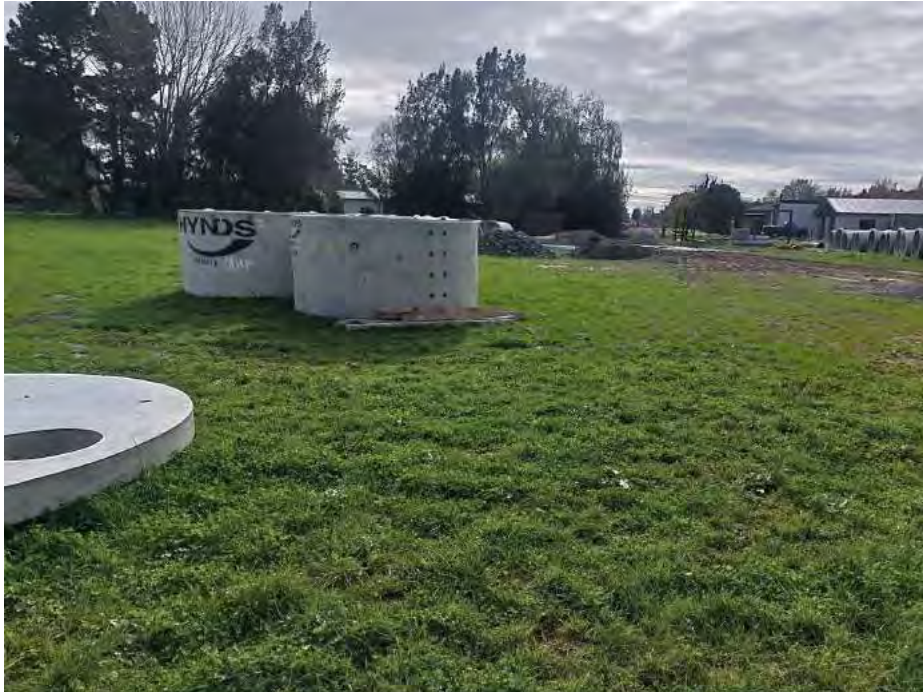
Plate D16: Looking northeast across grazing land. Note Trent Street towards the right-hand side of the photograph and the concrete pipes in the foreground.
