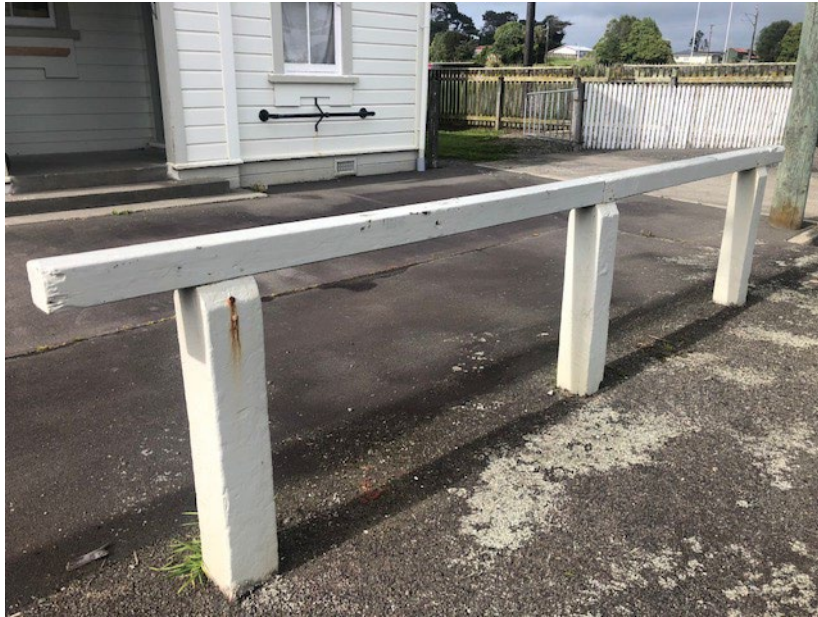
Figure 7 Note the hole through the rail in the middle of the closest span. Presumably the brackets beneath the windows of the post office, were also used as bicycle racks. (Photo: Rochelle Waugh, 26 September 2018)
