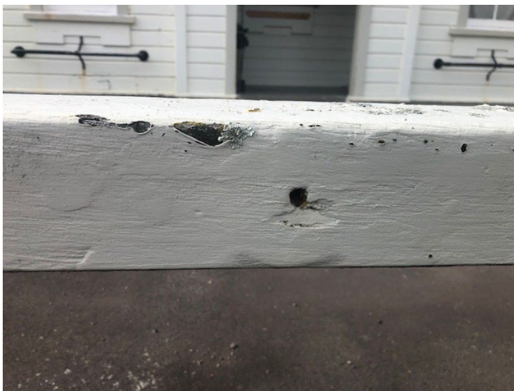
Figure 10 The hole in the rail – the purpose of which is unclear. The brown paint that was used for most of the life of the top rail, can be seen where the white paint has peeled back. (Photo: Rochelle Waugh, 26 September 2018)
