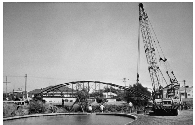
Figure 3 Installing the overbridge into its new location over the Makino Stream on 27 February 1978. (Source: Feilding Library photo: UTS:rr5: http://feilding.recollect.co.nz/nodes/view/16983 )
