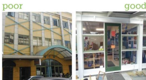
The two examples of external strengthening above contrast. The poor example (left) has cross braces (painted green) that run diagonally counter to the building's modulation. The good example (right) has a portal type bracing that fits with the door and window frame proportions and is painted the same principal white colour to de-emphasise it.
